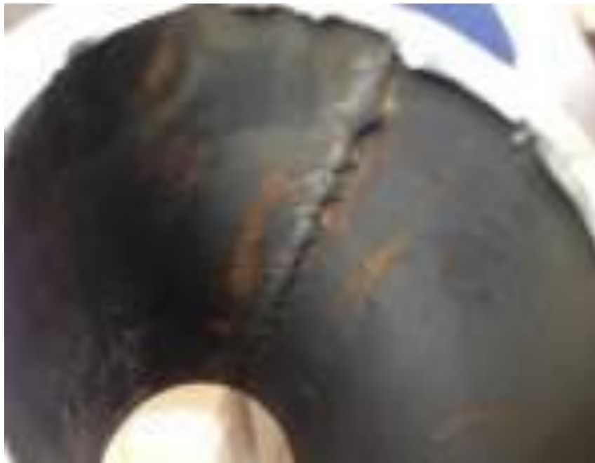
Fig. 6. Closed system recirculating water line treated for fifteen years with Polyamine Emulsion technology.
